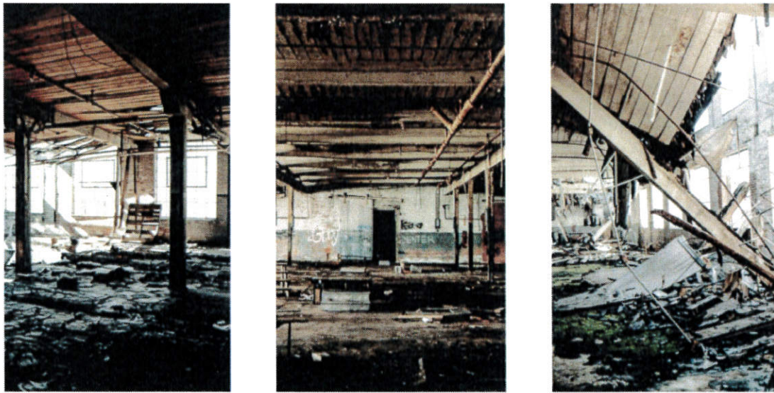
Figure 4 | Mill Conditions Prior to Recent Stabilization Efforts
